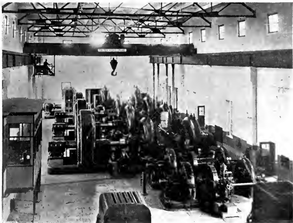
Interior of Power House showing 2 excitors, 3,500 h.p. direct connected units, and new 12,500 h.p. unit in background — Operating room to left, transformer gallery in foreground.
